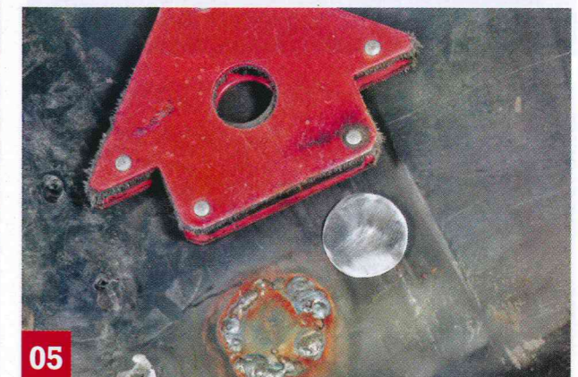
05 Access holes are filled and new ones cut. Use a welder's magnet to hold the fitted discs in place during welding
